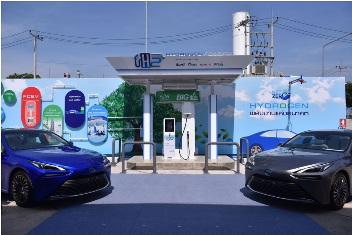
Figure 3.64. Prototypes of Fuel Cell Vehicle and Refuelling Station, Bang Lamung, Chonburi
