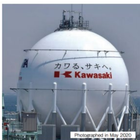
Figure 3.11 (a). Liquefied Hydrogen Storage Tank
